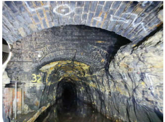
1790s brick lining giving way to rock-cut tunnel; the space on the left of the photo is an emergency adit originally dug to remove spoil and waste from the Nicholson tunnel.
